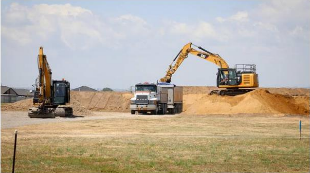
Diggers remove the stockpiled fill in Golden Sands in December. Photo / Andrew Warner
